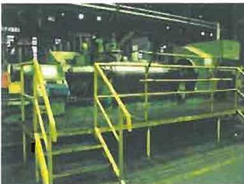
Cold rolling mill – MACHINE FOR GRINDING ROLLERS
