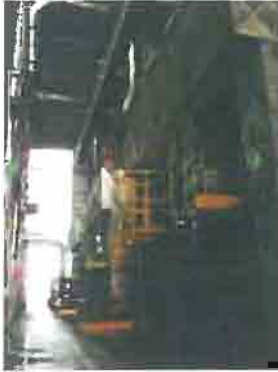
Power plant – STEAM BOILER
