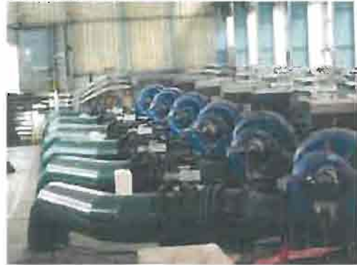
Power plant – PS OF RECIRCULATED COOLING SYSTEM OF BF2
