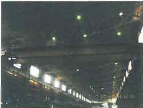
Tinplate Šabac – STRUCTURE OF TWO LEVEL RAIL CRANE D-1080
