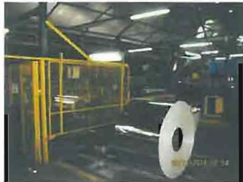
Tinplate Šabac – PAY OFF REEL NO.1 WITH MOVING PLATFORM
