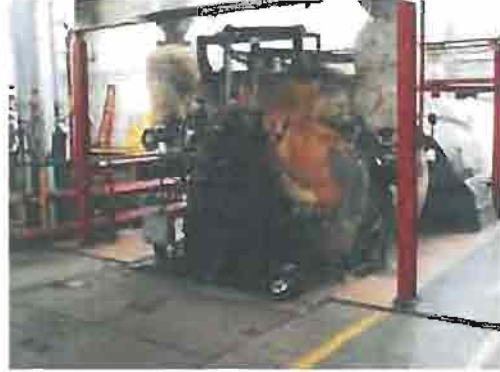
Power plant – TURBINA
